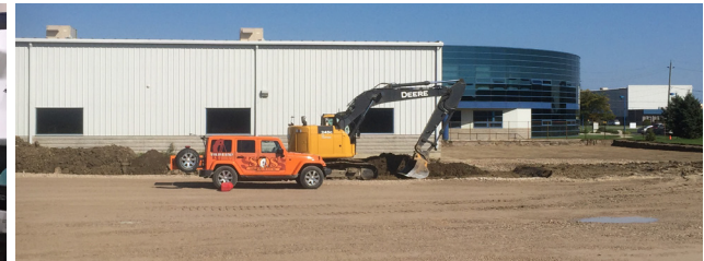
Construction has begun on the 50,000-square-foot expansion and is scheduled to be completed in February 2017.
